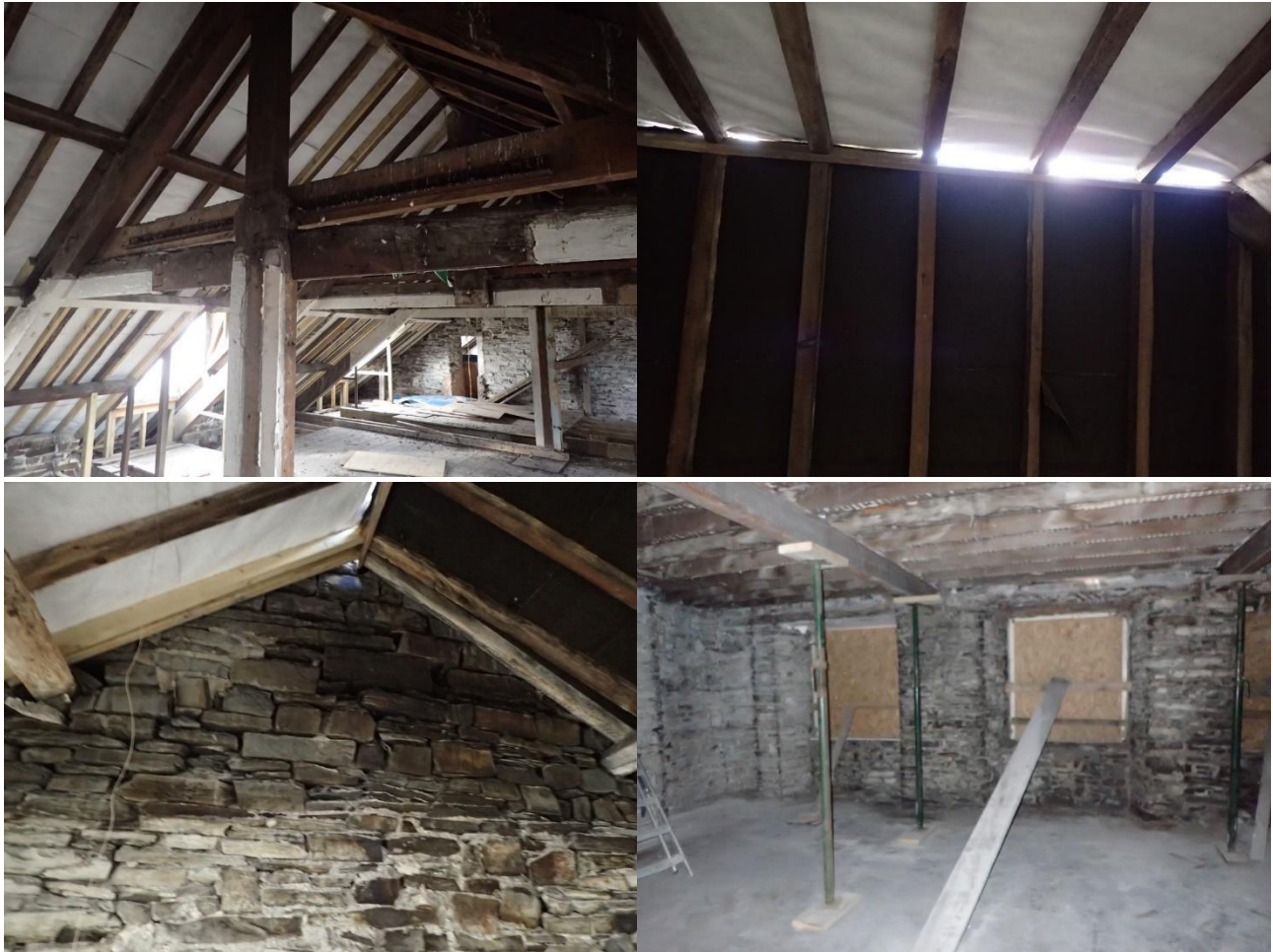
Internal photographs (clockwise from top-left): Upper storey; currently un-tiled ridge showing newer (white) membrane and older (black) bitumen membrane; ground floor; crevices in internal gable-end wall
